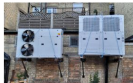
The units which have been attached to the rear of a High Street premises
